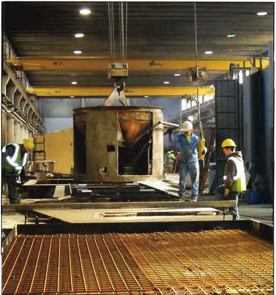
Workers pour the wall panels for the restroom facilities. In March, Carr Concrete will begin to ship the precast structures to various park and recreation locations in Nebraska, Iowa, Kansas and Missouri.
