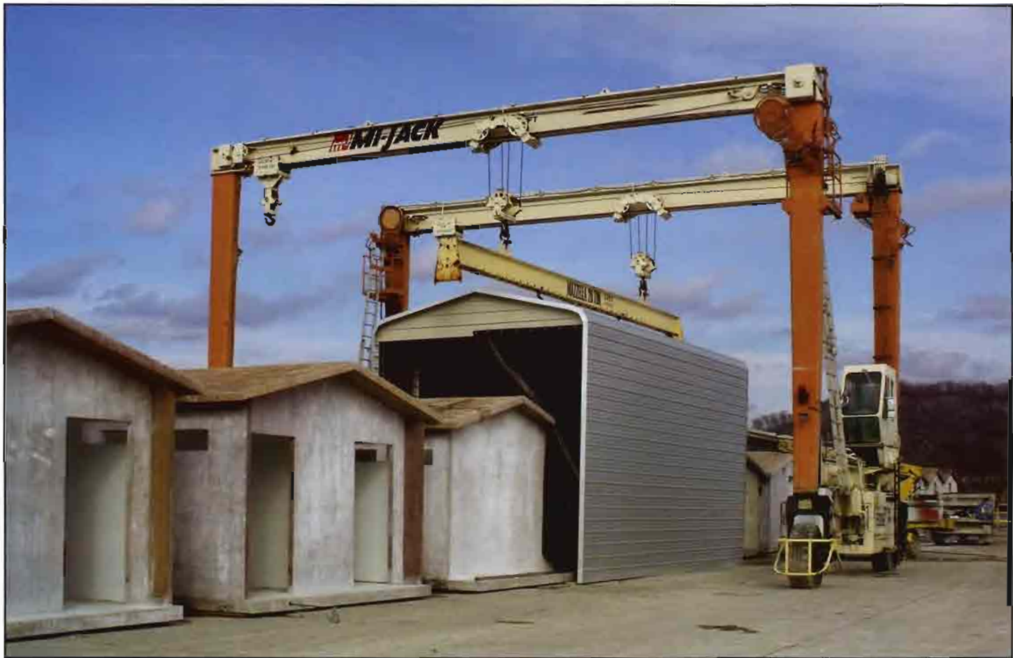
The restroom facilities contract includes all finishes, plumbing fixtures and roofing. In order to maintain the aggressive production schedule throughout the winter, Carr Concrete utilizes a mobile garage. The schedule has also permitted the company to operate two shifts, allowing them to keep up with the project along with their other building production work.
