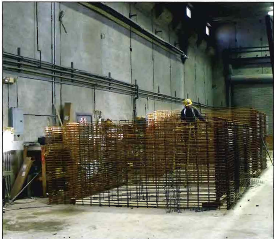
Carr Concrete is also producing 265 box culverts for a section of Corridor H in Grant County under construction by Vecellio and Grogan, Inc., Beckley. A worker assembles the rebar for the box culvert.
