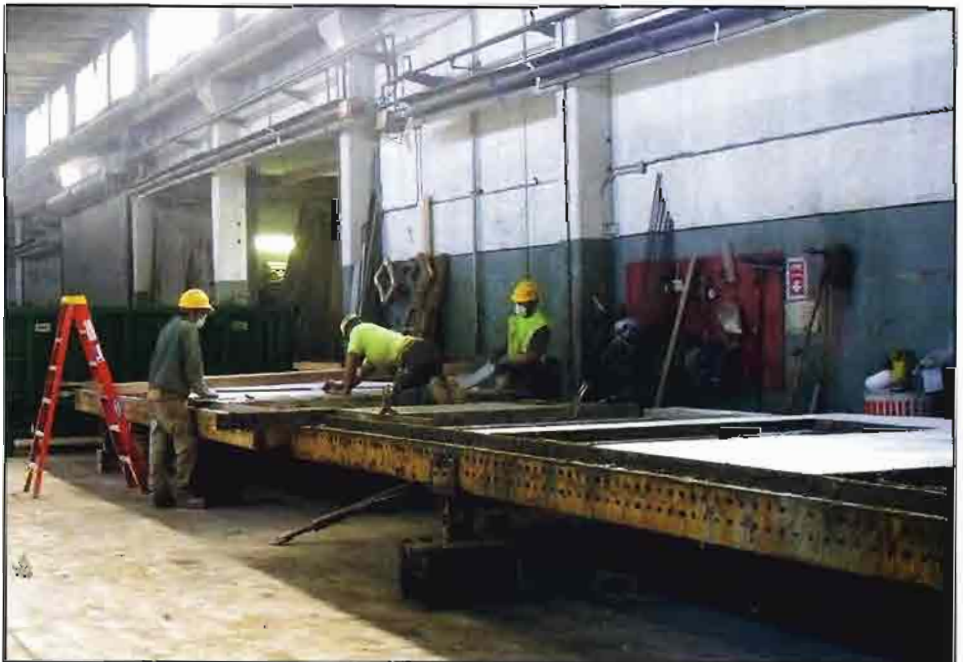
Each of the 130 facilities has one of 13 designs. Size, layout, materials and finishes vary. Workers apply woodgrain, stone and other finishes to the exterior of the panels after they are poured.
